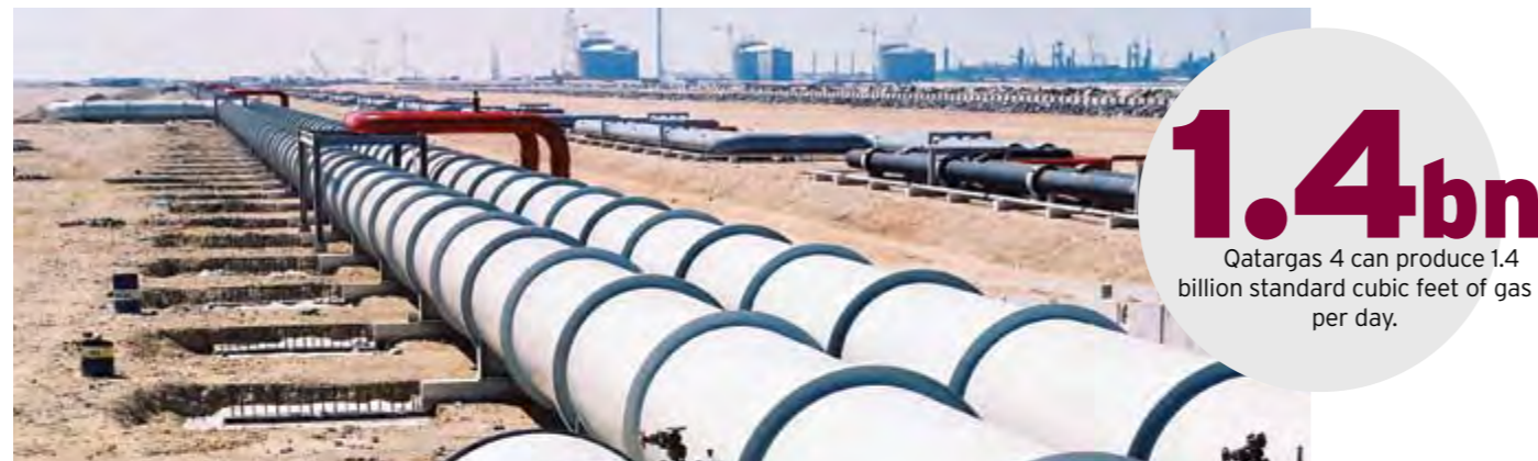
The upstream platforms and infrastructure consist of three unmanned platforms (each containing 11 wells) and two sub-sea pipelines, which are shared with Qatargas 3.
